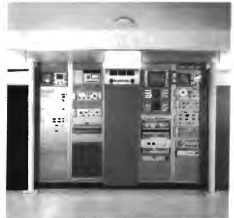
Control and monitoring racks. Center unit is parallel control cabinet for total system aural and visual output, and for automatic exciter switching. Other racks mount audio and video input monitoring and remote control equipment. System layout was designed by Transmitter Supervisor Bill Stevens.
